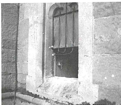
26 May - 19th C. leaded window, wrought ironwork and stonework damaged
