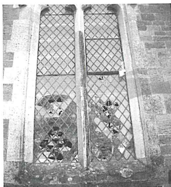
9 June - Two 19th C. leaded windows damaged -
